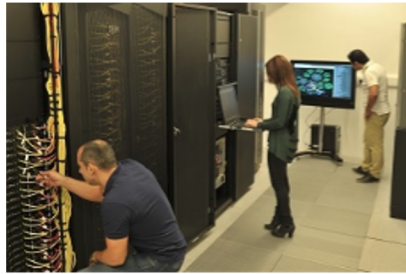
High-Performance Computing Facility
