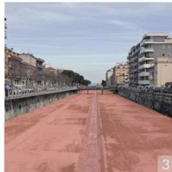
3 Albula stream completely cemented, does not allow water absorption in case of flooding.
